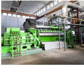
Diesel Electrical Generator
