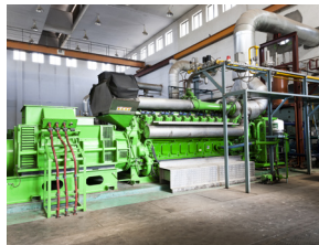
Diesel Electrical Generators
